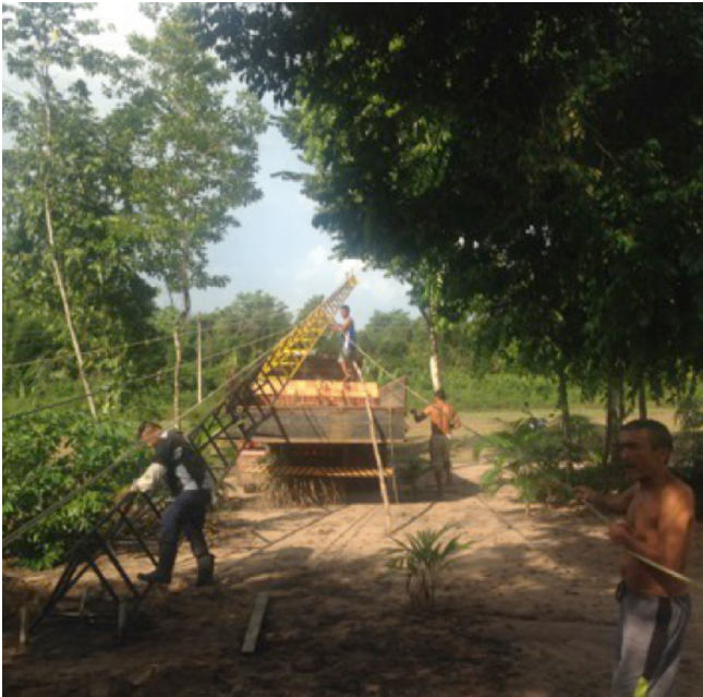
Figure 2. Installing the tower that carries the internet antenna in the center of the community.
