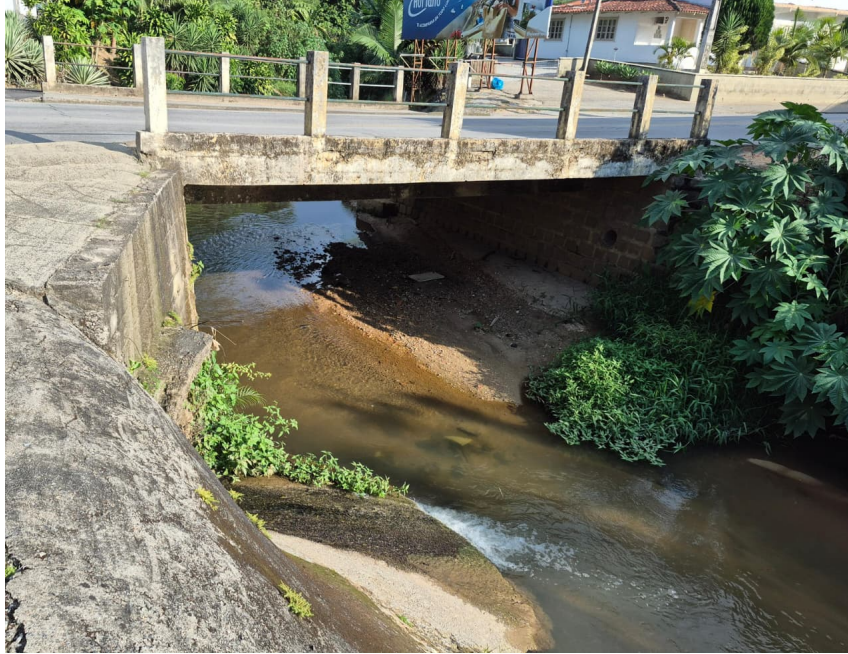
Figure 1. Lateral view of Bridge 2 from the river margin, showing the bridge structure and surrounding environment at the field deployment site.
