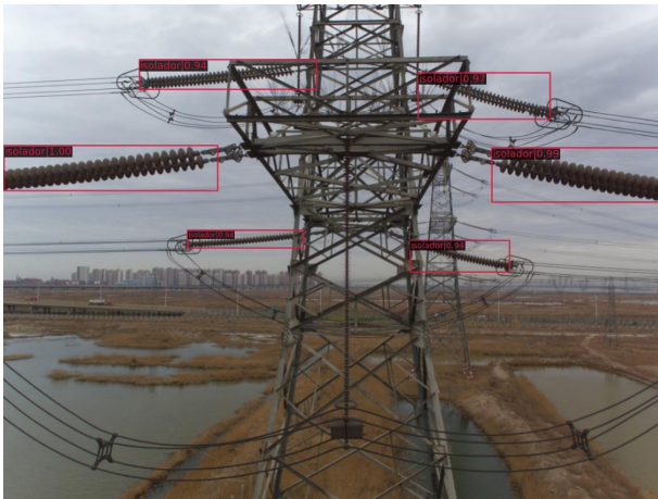
Fig. 9. High-Voltage Power Line Multiple Insulator Detection Example.
