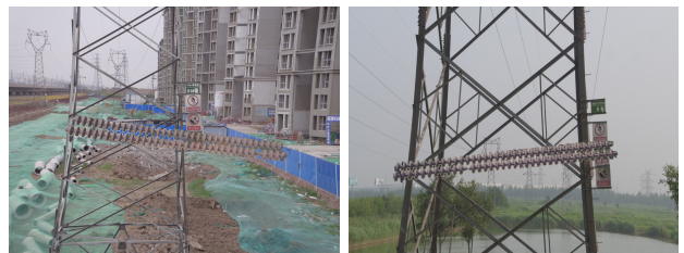
Fig. 2. Defective Power Line Insulator Example.
