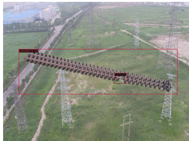
Fig. 8. High-Voltage Power Line Insulator and defect Detection Example.
