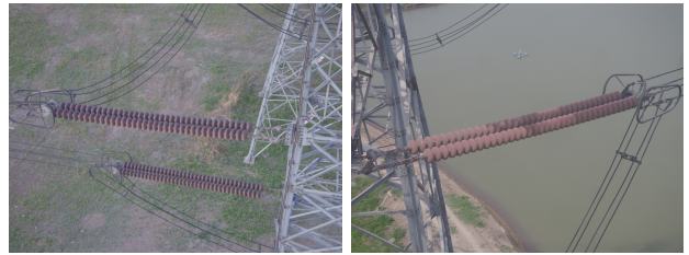
Fig. 1. Normal Power Line Insulator Example.
